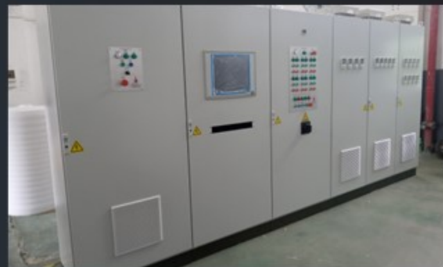
以PLC和HMI为基础的E-smart控制系统 PLC + HMI based Control Panel
